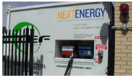
Figure 1: CEF's Biofuel and Emissions Fluids Dispensing Station
